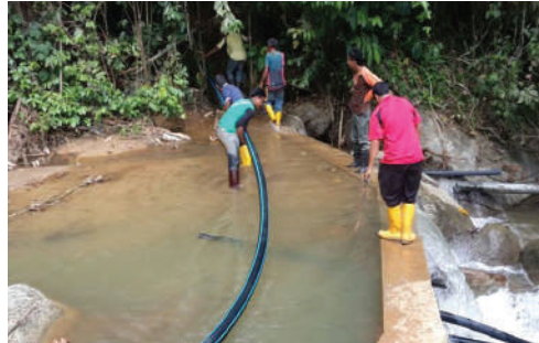
Image 6.20 Water Supply Through Gravity Feed System
